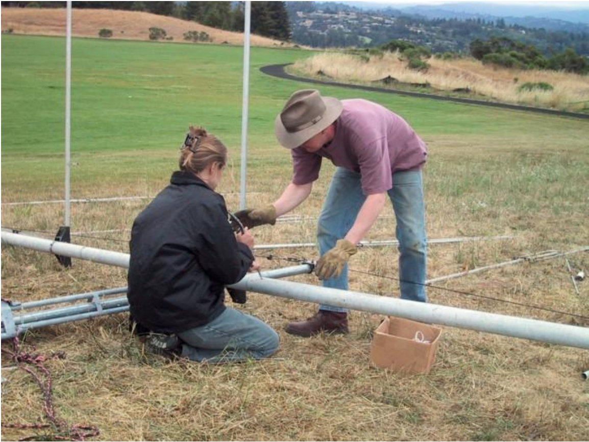
Steve Petersen, AC6P and Heather Levine work on assembling the HF beam. Note jogging track in background.
